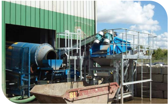
OPS Drainage Treatment Plant
